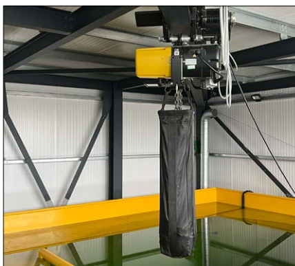
Steel hoist can be used for equipment anchoring and emergency diver recovery.
